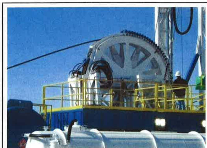
Wheel-based injectors offer less pull than traditional injectors, but need less maintenance, which makes them well-suited for drilling shallow wells. Many companies say that is where coiled tubing drilling shines.
